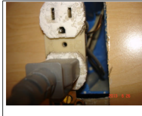
One of several plugs not secured and covered.
