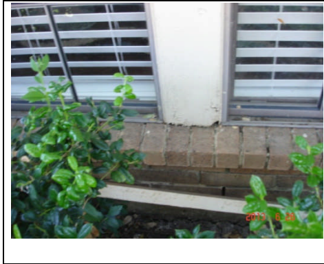
Rotted siding at dining room window
