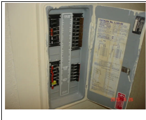
FPE stab-Lok installed in bathroom
