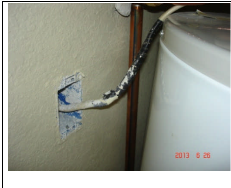
220 wires improperly spliced outside of junction box.
