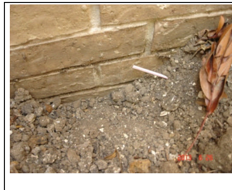
Soil 4 inches or more above foundation wall.
