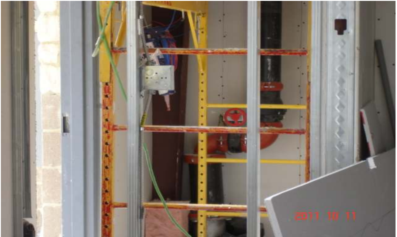
Fire sprinkler valve system has been installed.
