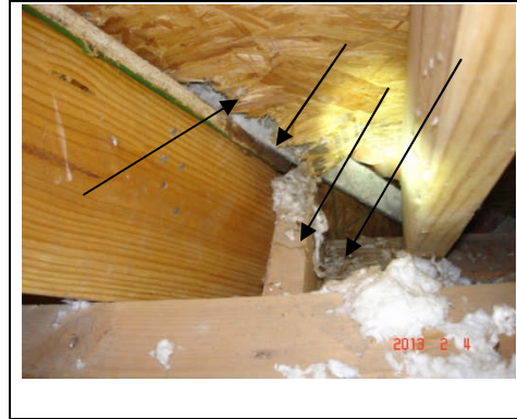
Damaged roof decking over office with evidence of water in attic
