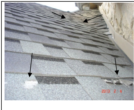
Damaged shingles over office
