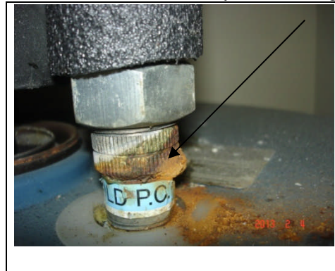
Water supply connection for water heater, corroded.
