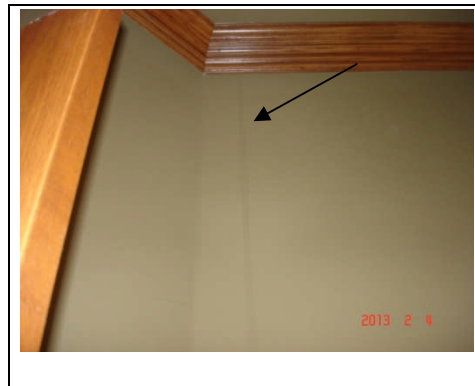
Water stain in office directly below damaged decking
