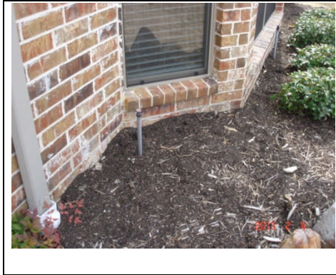
Mulch needs to be lowered around foundation.
