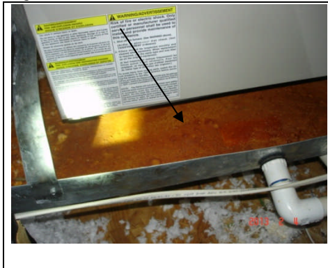
Evidence of clogged primary drip lines.
