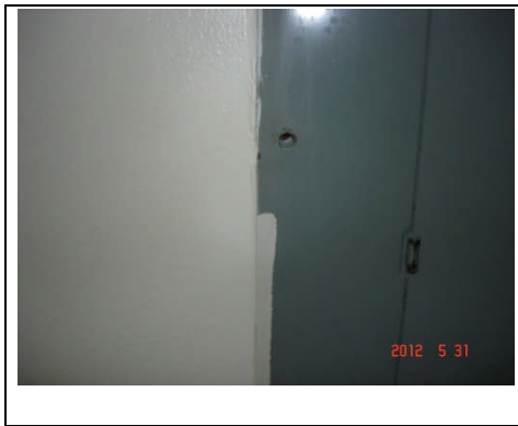
Fastener missing on breaker panel.
