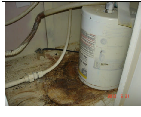
old water heater rusted and water stains under sink
